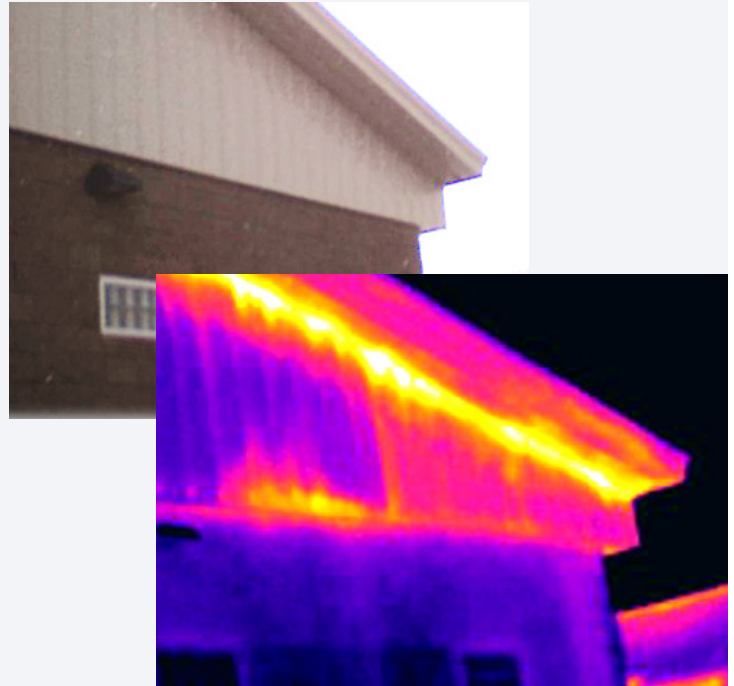
HUMINT inspection report included infrared camera images notating the "dripping" warm pattern indicating air leakage
